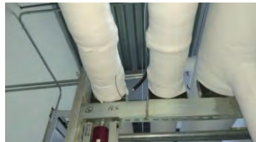
Cold water flow meter detector
